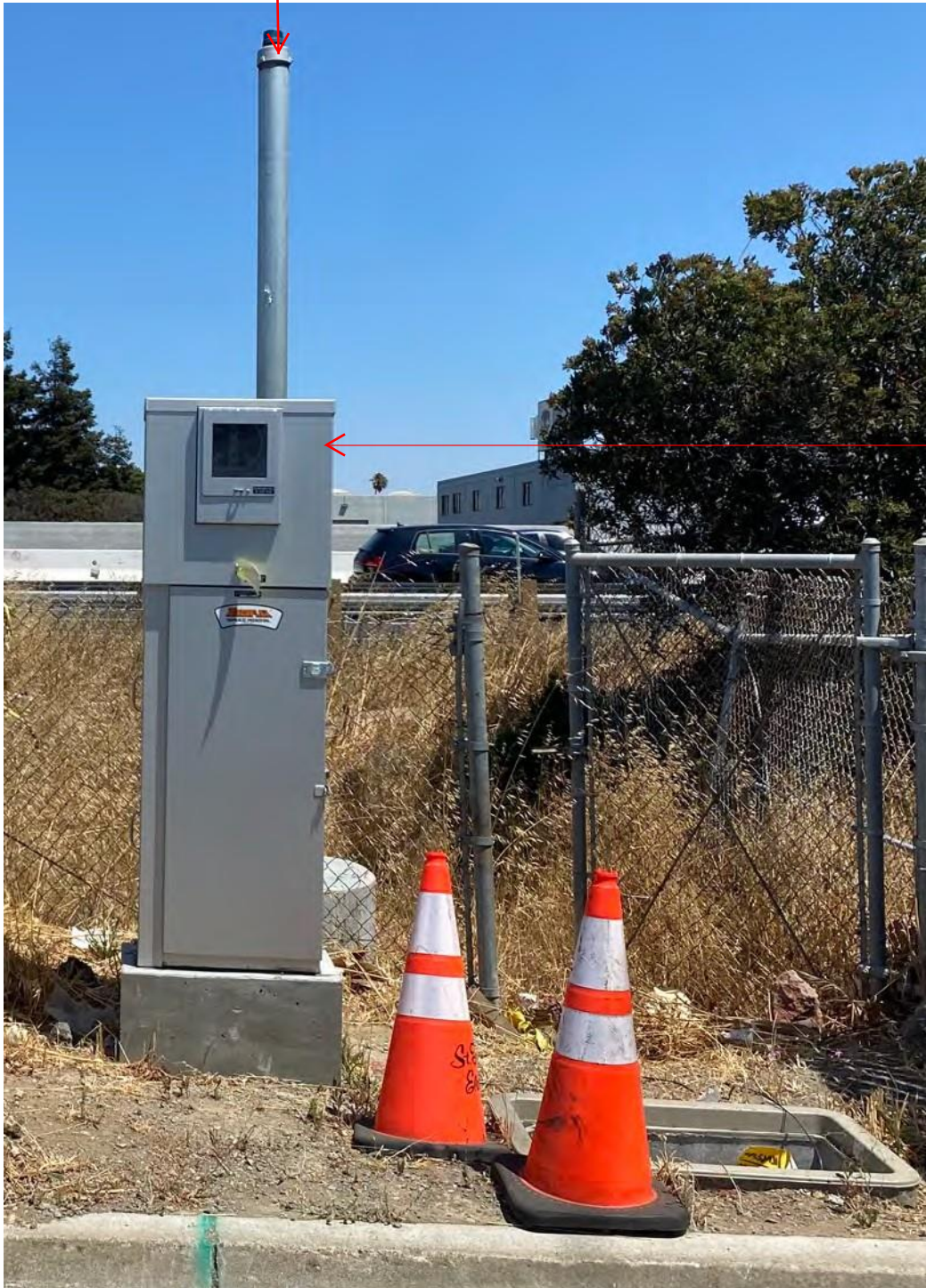
TOLLING ITEM #10: TYPE III-AF SERVICE EQUIPMENT ENCLOSURE NO. T17100
